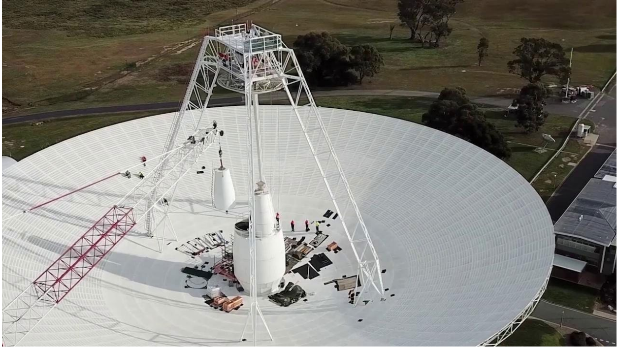
Crews conduct critical upgrades and repairs to the 70-meter-wide (230-foot-wide) radio antenna Deep Space Station 43 in Canberra, Australia. In this image, one of the antenna's white feed cones (which house portions of the antenna receivers) is being moved by a crane. Credit: CSIRO
